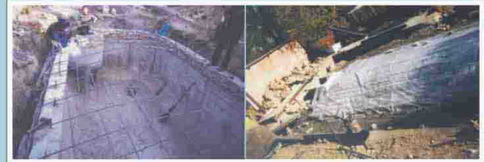
Erection of the dome is one of the most difficult stages of construction
