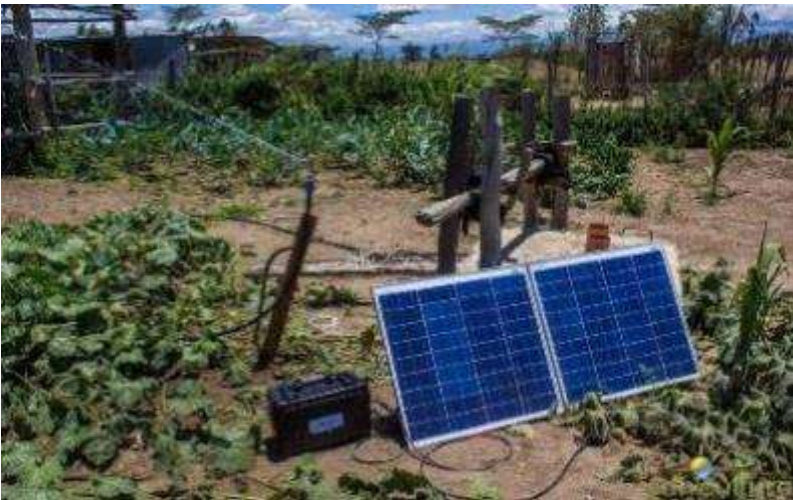
Solar powered water pump
