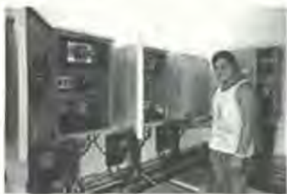
Solar electricity plant at Tuvalu. Photo: Pene Lefale
