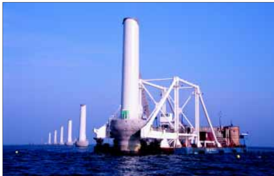
Placing the foundations in the shallow water of Middelgrunden. Photo by Mads Izmodenov Eskesen
