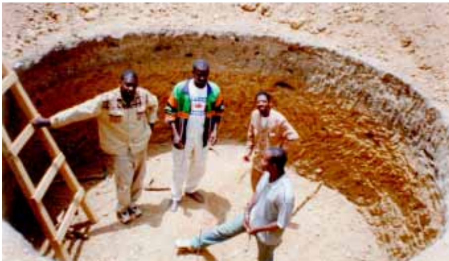
Digging a hole for construction of the digester of a family biogas plant. The Mali Folkecenter is the coordinator of this project, working in cooperation with the Malian Rural Polytechnic Institute. The project will consist of five installations, of which two have been completed. Funding is from the Global Environment Fund (Small Grant Program) of the UNDP.
