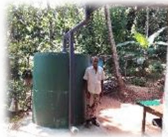
Roof rainwater harvesting.
