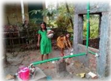
Rainwater Harvesting System
