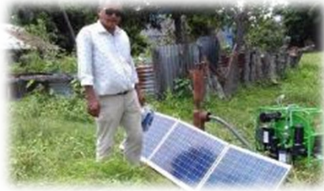
SF2 Solar Water pumps
