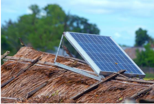
Solar Home System
