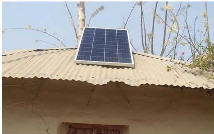
Solar Home System
