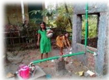
Rainwater Harvesting System
