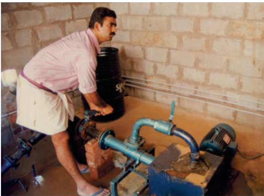
Small hydro system in Kerala, India.
