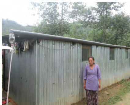
Rain water harvesting set up in the roof of Rupa's house
