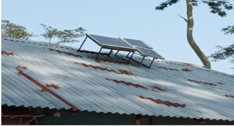
Solar Home System in Mathbaria
