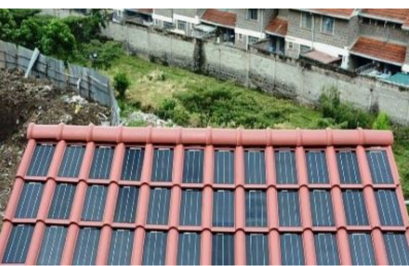
Solar PV roof
