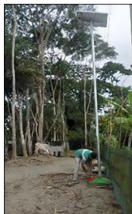
Solar powered street light.
